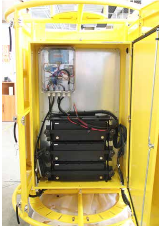
The expandable battery rack ensures uninterrupted operation with different configurations.
